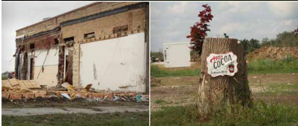
Silos remain twisted and torn and buildings remain damaged weeks after a tornado hit Greenfield. Support for the community has come from near and far. Photos: Steven Johnson
